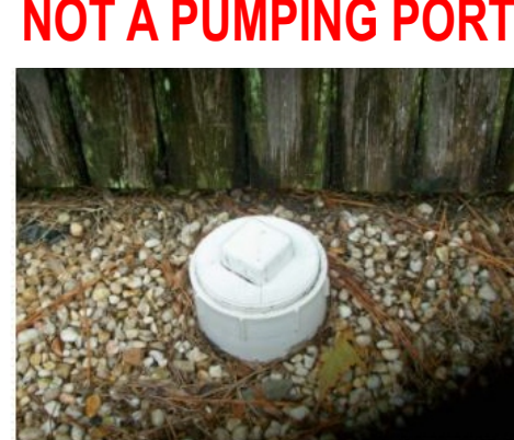
Inspection Port - Not A Pumping Port
